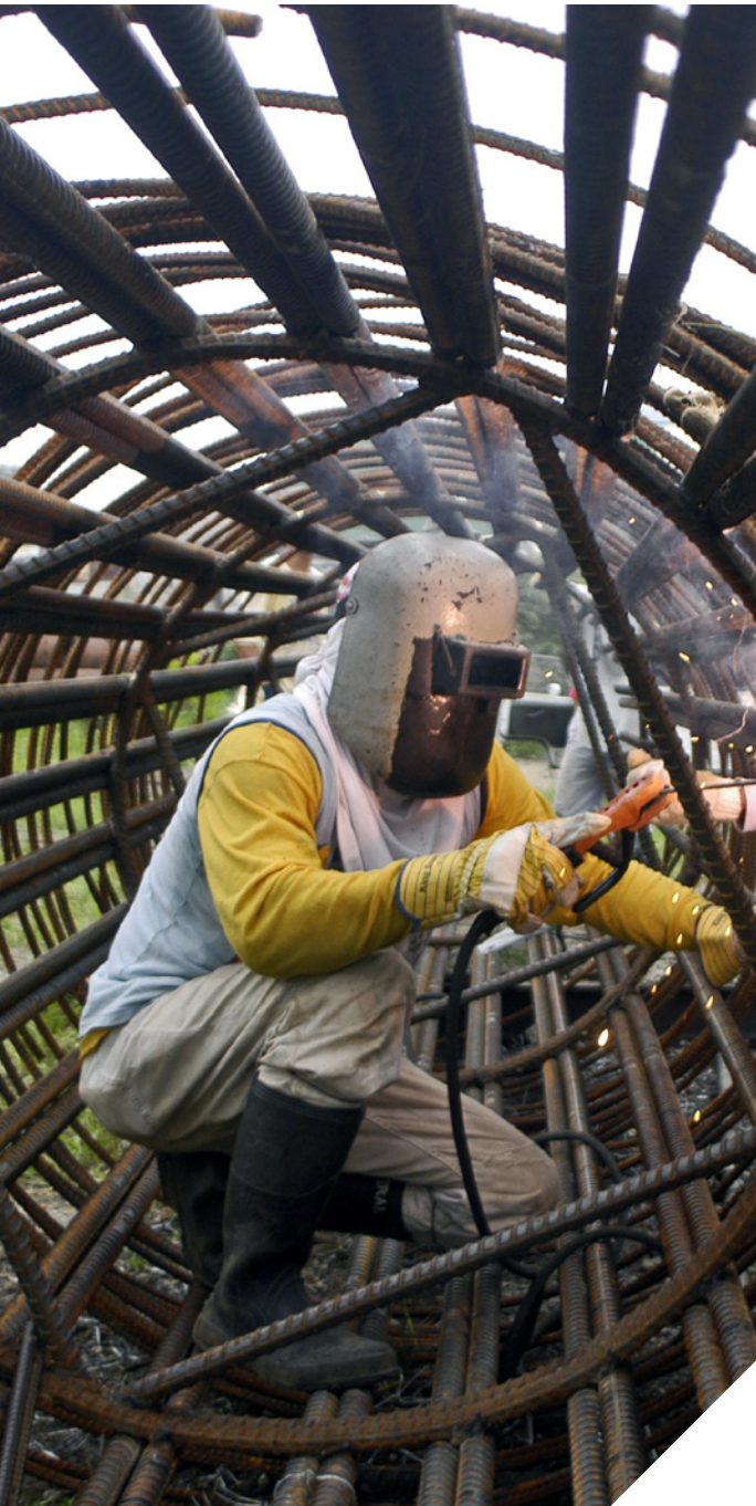
Man welding a large reinforced steel tube in the Philippines. - Nonie Reyes / World Bank Photo Collection
